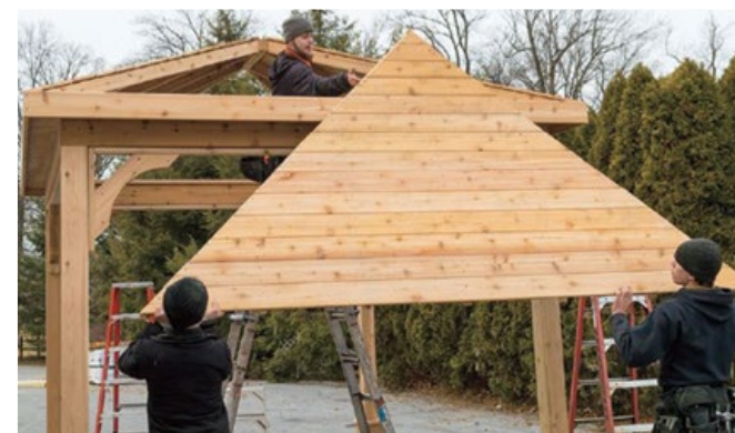
A) We notch the tops of your 6x6 posts 1 1/2" on both sides to fit your 2x8 beams, and B) we notch your 2x8 beams 1 1/2" deep to fit your 2x6 rafters
